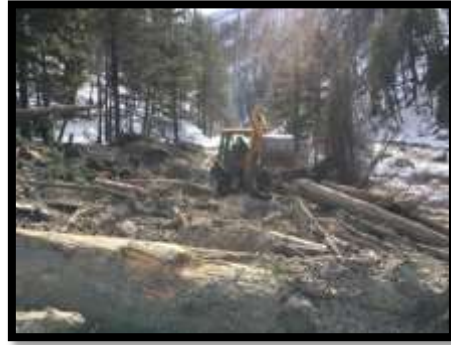
Cleanup after landslide onto East Fork Road
