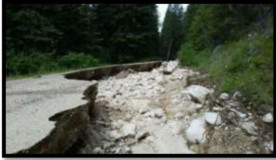
Washout of Lick Creek Road
