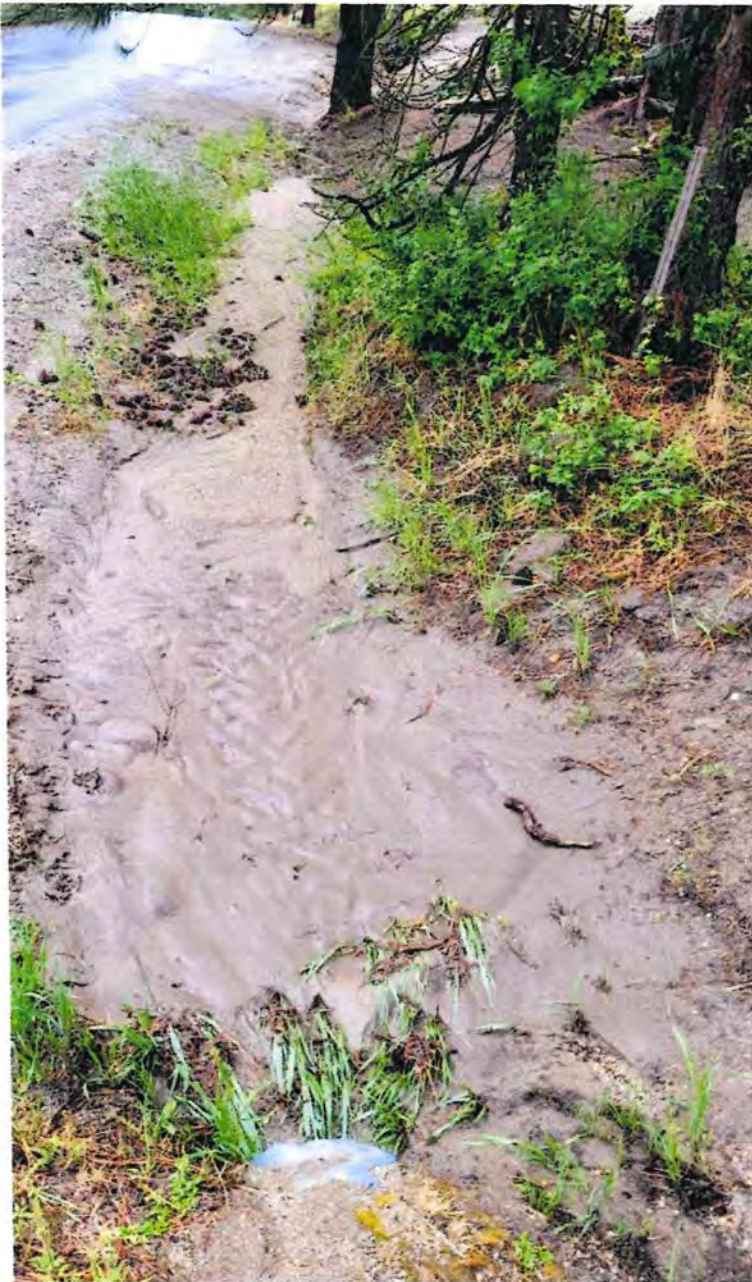
Picture 3 a and b: excavation silt blocking ditch
